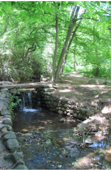
Runoff from surrounding properties damages Dumbarton Oaks Park's historic landscaping.
