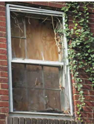
The poor condition of Chesapeake House invites further vandalism.
