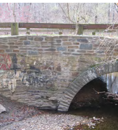
Vandalism poses ongoing challenges for the NPS maintenance staff.
