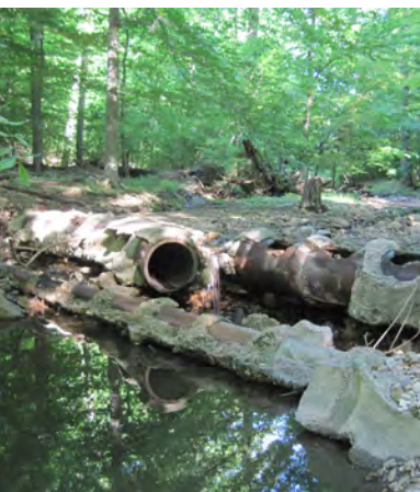
Soil erosion exposes pipes buried near streams and threatens park roads, bridges, and trails.
