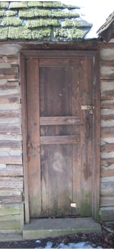
The cabin’s walls are deteriorating, and there is a hole in the locked door.
