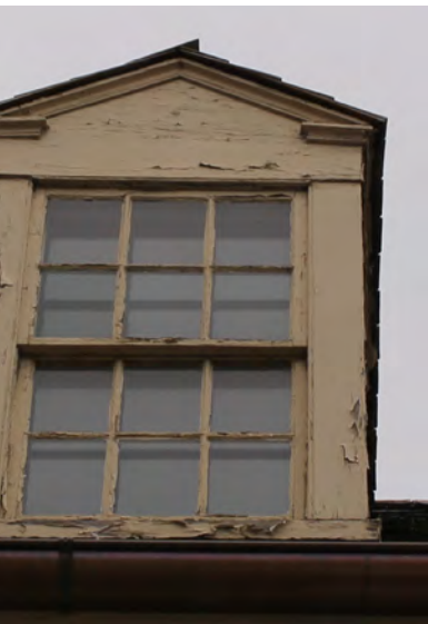
As with any historical building, the house has ongoing maintenance needs.
